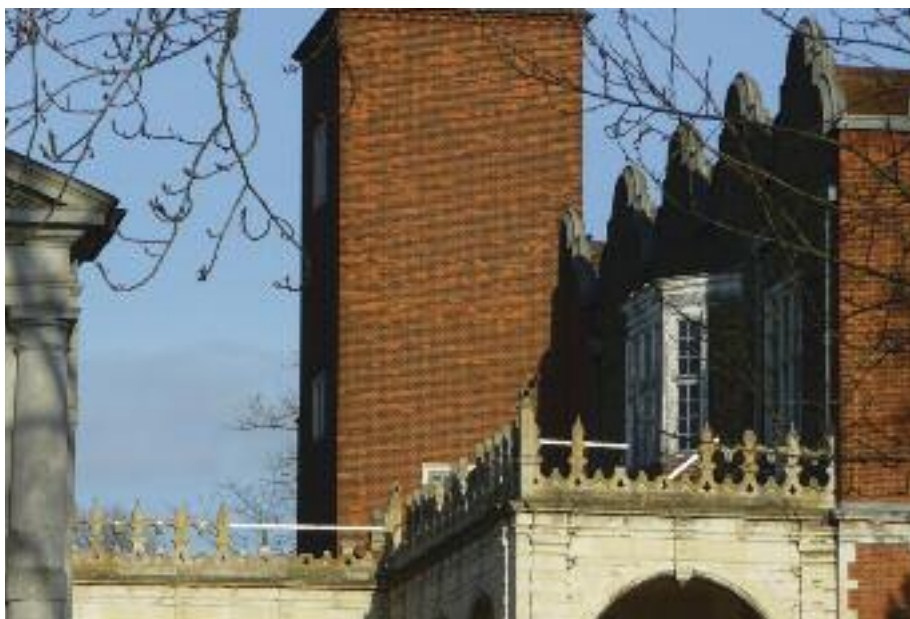
Holland House in January 2018, with finials missing
